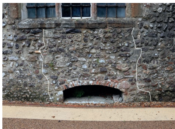
Fig 46. Patch of inserted walling above arched recess showing it is secondary to the original (Norman) fabric. Photograph: authors.
