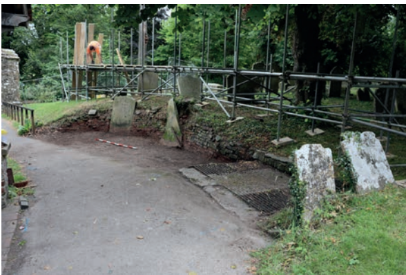
Fig 11. View in front of south porch before 2019 excavation showing mid-twentieth tarmac path and nineteenth-century niche (with headstones) constructed to display the foundations of the Anglo-Saxon apse. Photograph: authors.
